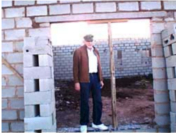
Jim in the half-built hospital. The far wall is the one that fell, killing two students.
